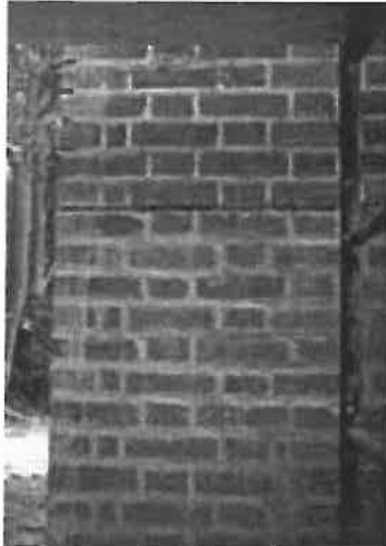
This 19 th century brick has been damaged by improper grinding of joints and sloppy application of mortar.
