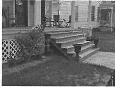
New wood steps have been installed at this East Main Street porch, maintaining its historic character.
