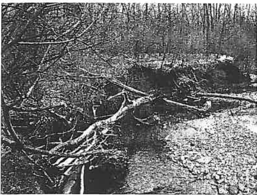
Bank Erosion along Muddy Creek
